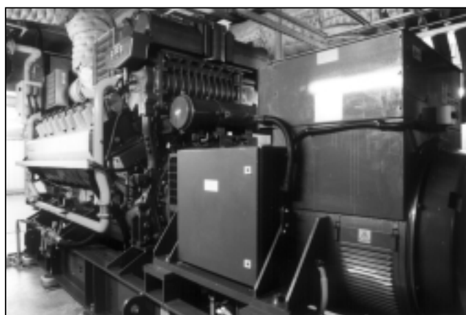
One of six 18 cylinder natural gas engine powered Cummins QSV91G CHP Generating sets for an installation producing 1750 kWe and 2000 kW of heat per set.
