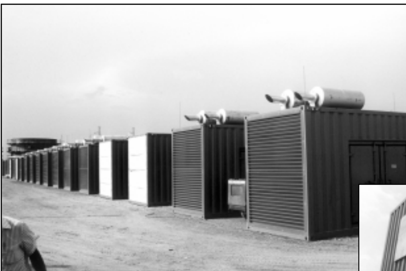
Multi-set installation with 28 x 1 MW generators would produce 20 MW continuous output.
