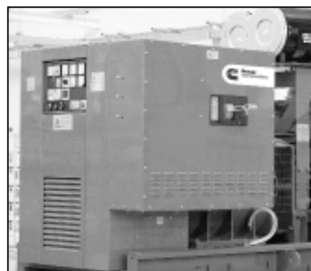
Set mounted 1000 ampere circuit breaker.
