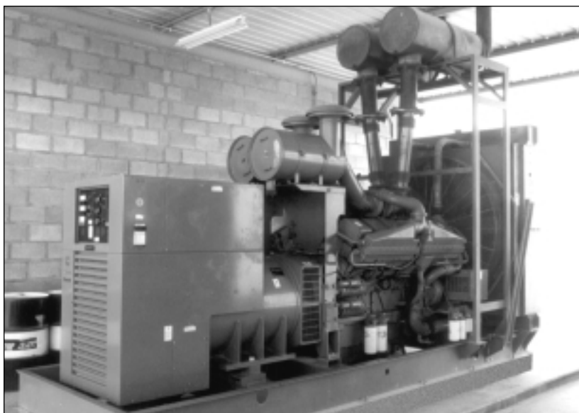
Model 512 DFGB (640 kVA) in a typical hot climate installation.
