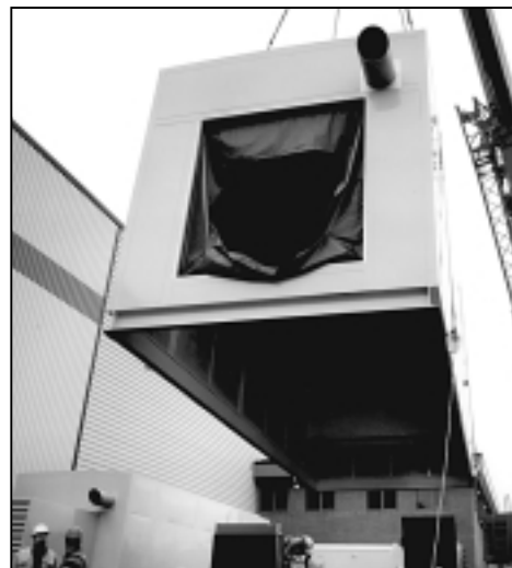
Fig. F10 Drop over super silenced enclosure for 2 x 1000 kVA standby generators.
