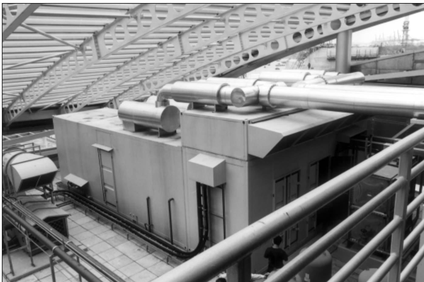
Twin 1875 Kva generating sets with Cummins QSK60G3 engines installed on a 10 story roof top installation for Data Computer Centre. Silenced to 75 db(A) at 1 m, each set weighed 26,000 kg with a control panel container weighing 700kg. Congested City Centre meant the installation had to be carried out at night.
