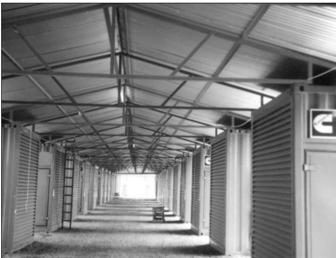
Multiple low voltage generator installations.
