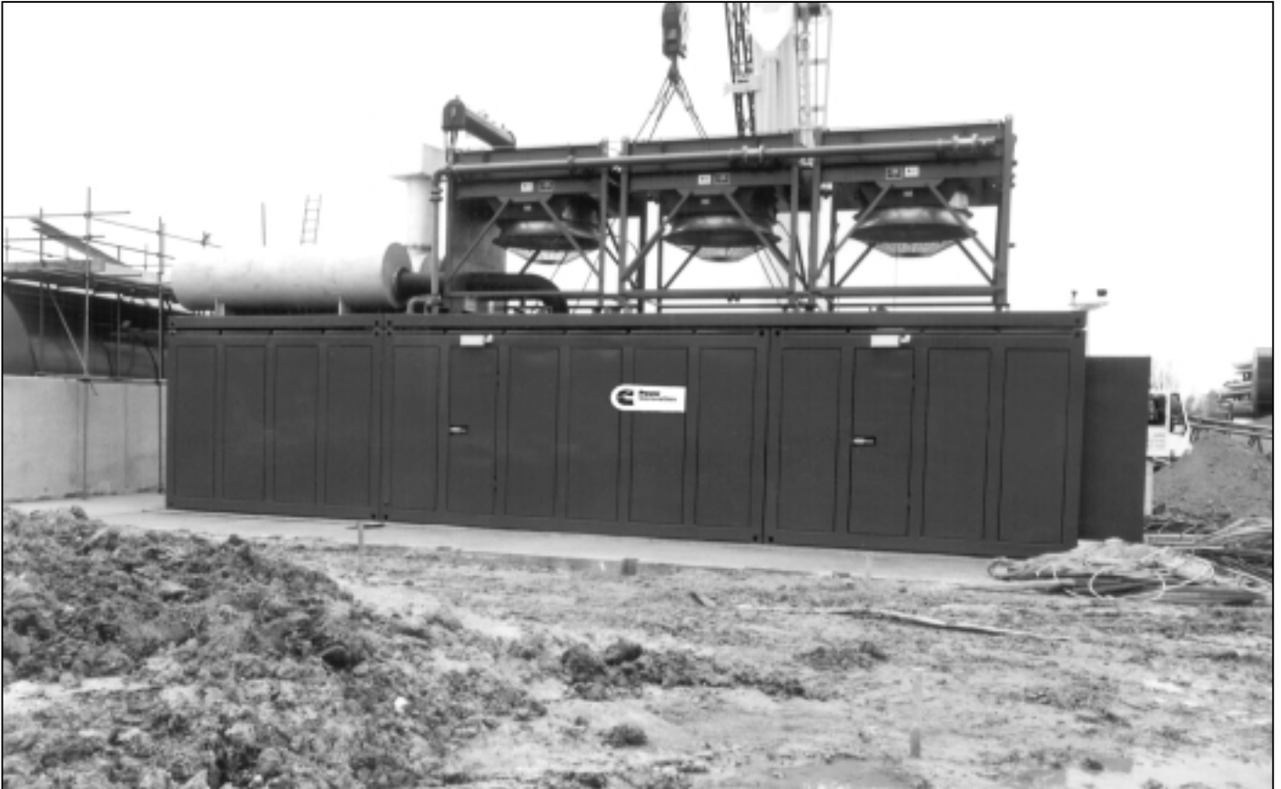
Complete installation with roof mounted radiators and exhaust system for 1750 kW gas powered set.
