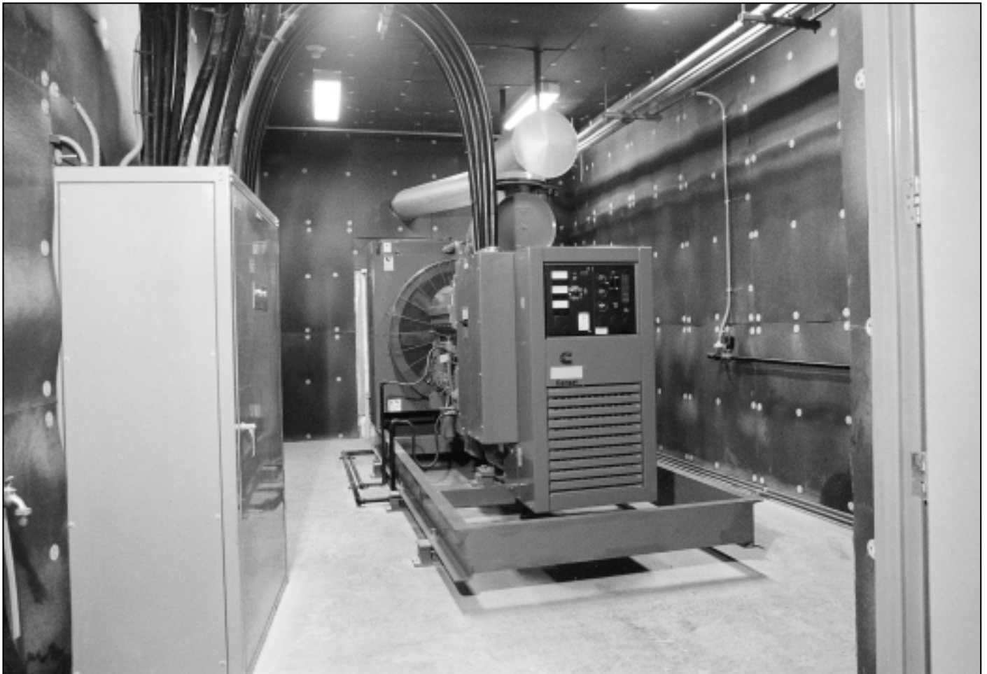
Terminal box on Control Panel for transferring output to floor mounted auto transfer cubicle for a 625 kVA set.
