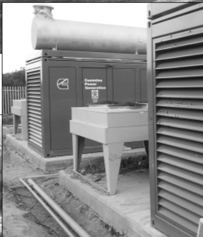
Fuel piping and auxiliary cabling runs.
