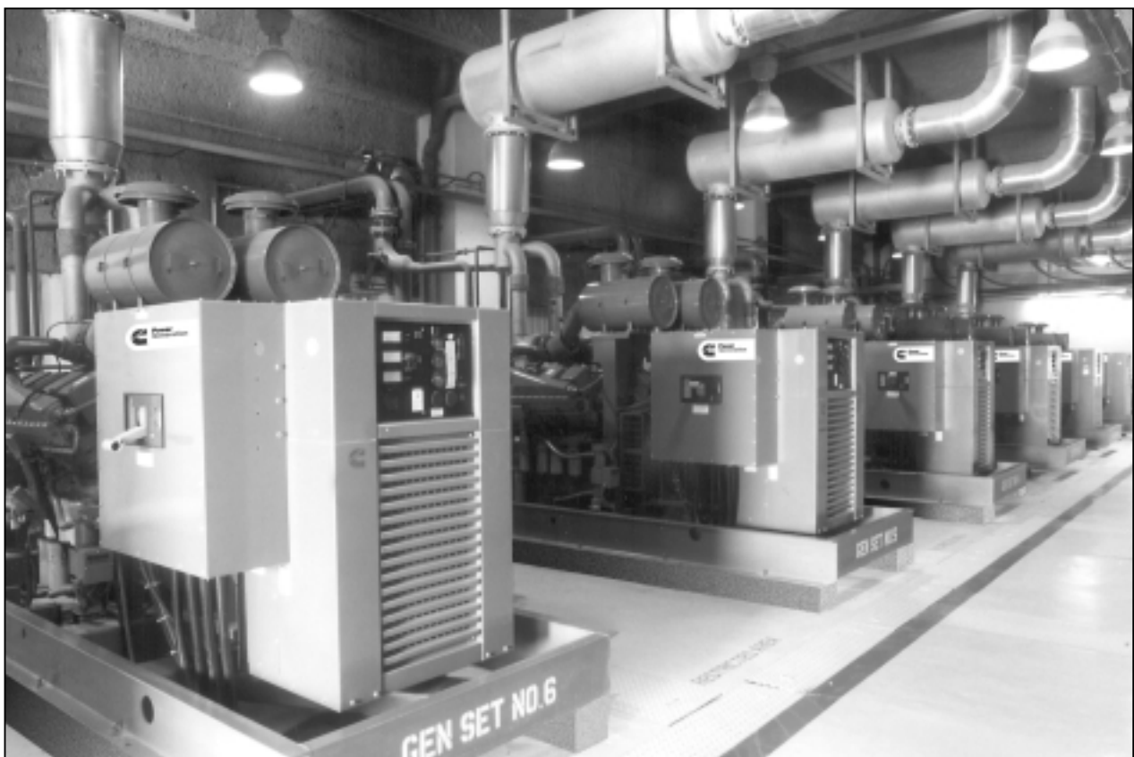
Seven 900 kVA sets working in parallel using the PCCP control system for a major soft drinks bottling factory in the Middle East.
