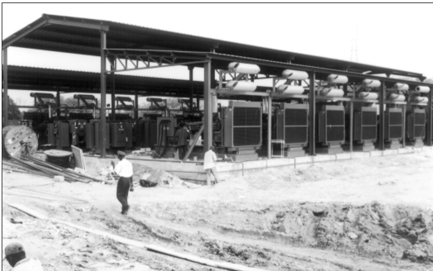
High voltage multiple generators operating in isolation from any external supply.
