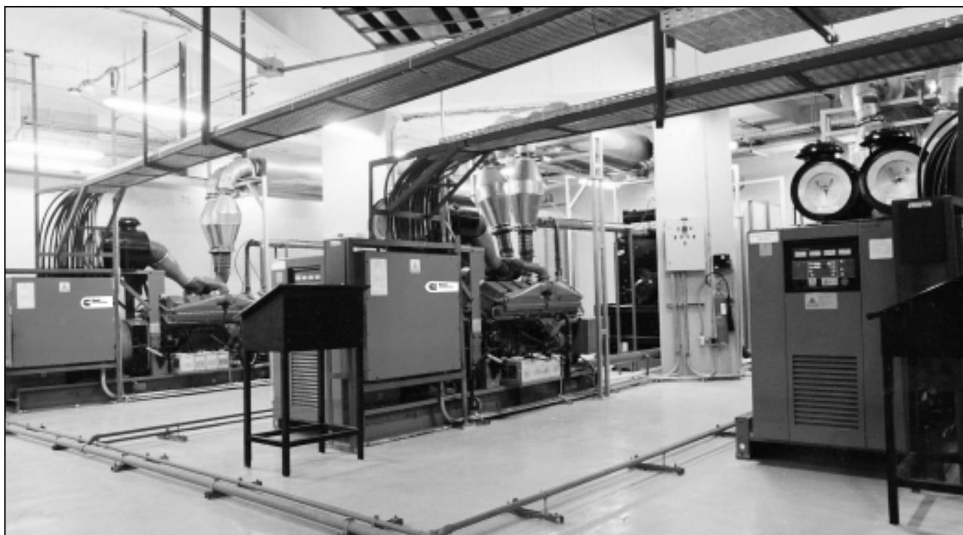
Three 1 MW standby sets powered by KTA38G4 engines installed in a hospital with catalytic converters to reduce exhaust emissions.
