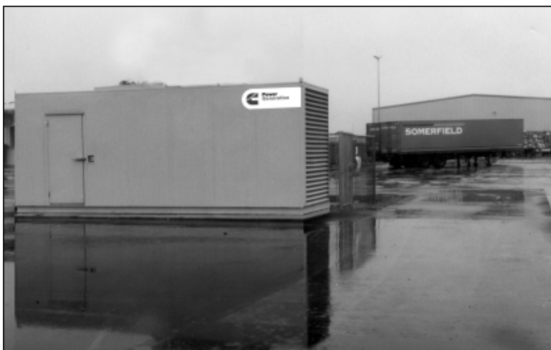
Fig. F3 Silenced enclosure for 500 kVA meets 75dB(A) @ 1 m.
