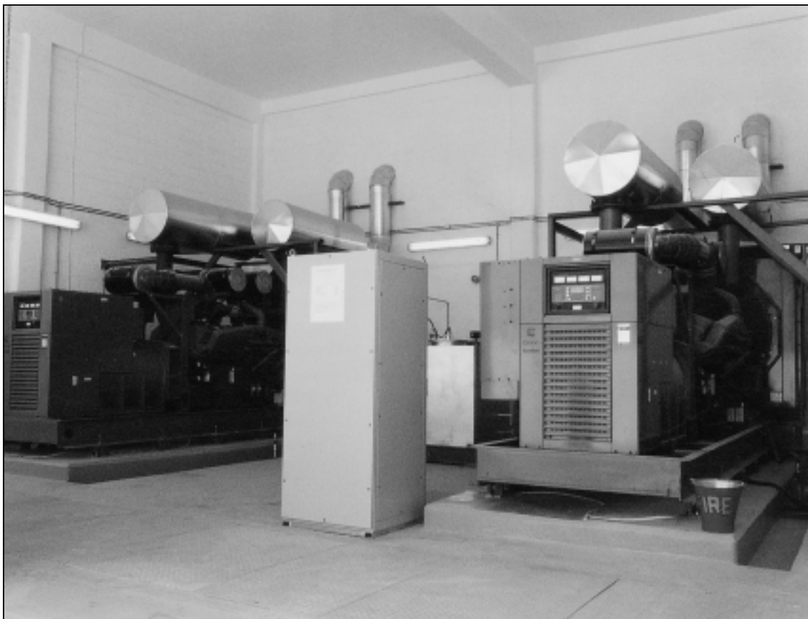
Generators that operate independently of an external supply and in parallel.
