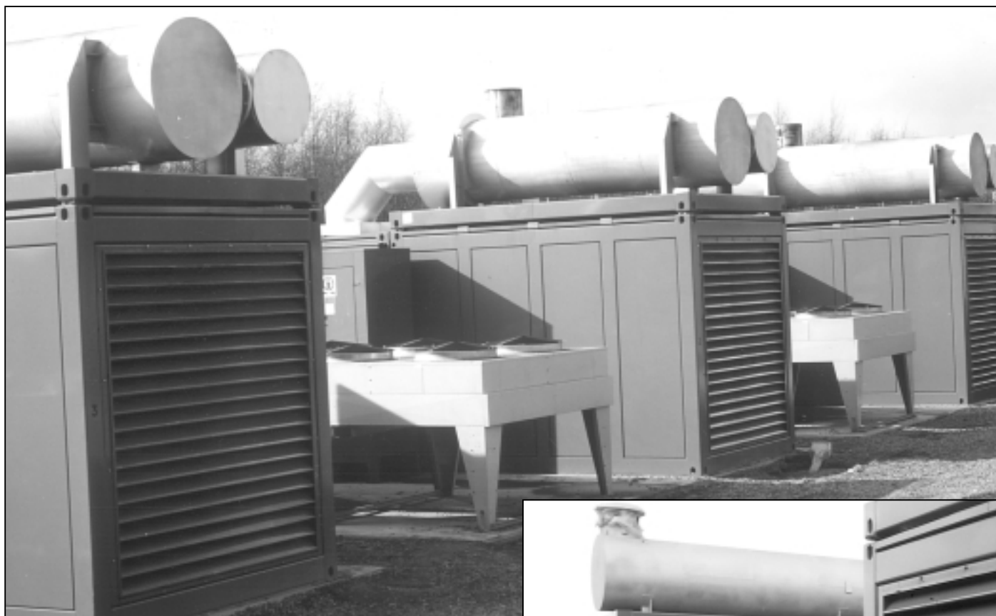
Containerised, 1.57 MW HV sets used for peak lopping duties with horizontal external cooling radiators. Whole installation silenced down to 75dB(A) at 1m and inaudible at around 50ft.
