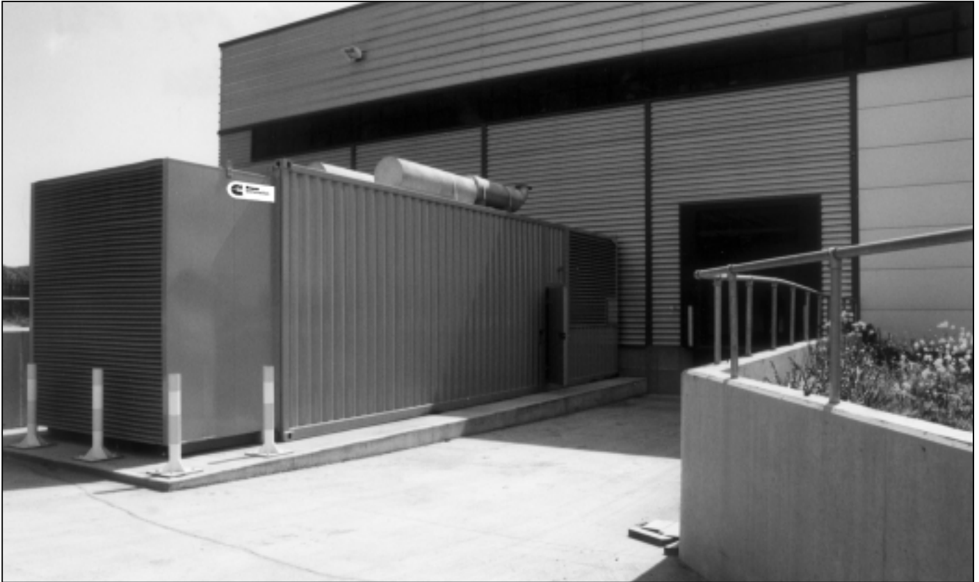
12m (40ft) silenced container enclosures a 2000kVA standby generator. Low noise level allows close proximity to building for short cable runs.
