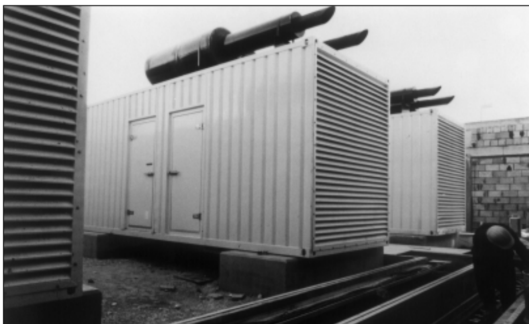
Three Cummins 1000kW silenced generators. Method of concrete foundation eliminates laying a large concrete platform over the whole area – saving costs. Method can also be used on roof top installations where point loading is sometimes necessary.
