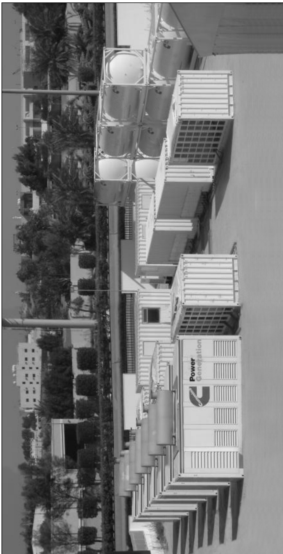
Example of 5 MW Power Station Module with 7 x 1 MW Generating Sets. Note 6m (20ft) container packs for transformers, control and switchgear. Stacked on right hand side are 22000 litre fuel tanks in 6m (20ft) packages.
