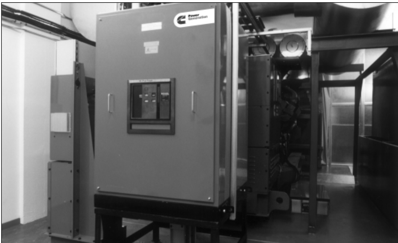
Free standing motorised circuit breaker.
